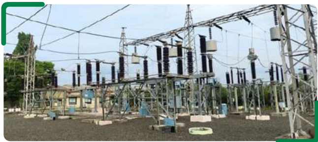
Substation augmentation at Talegaon, Wardha | MH | 132 kV
