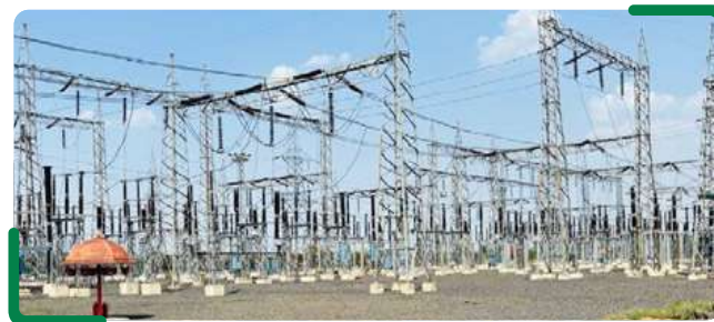
Substation augmentation at Umred, Nagpur | MH | 220 kV
